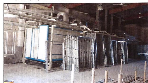
* OVEN POWDER COATING LINE SYSTEM
